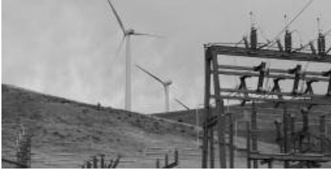
Leaning Juniper Wind turbines overlooking Columbia Basin Electric Cooperatives Alkali Substation.
