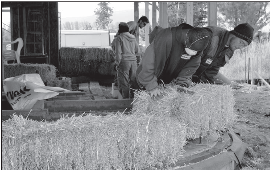
Volunteer Maxwell Danlogo, left, and Izaak Edvalson install straw bales on rebar to provide stability.
