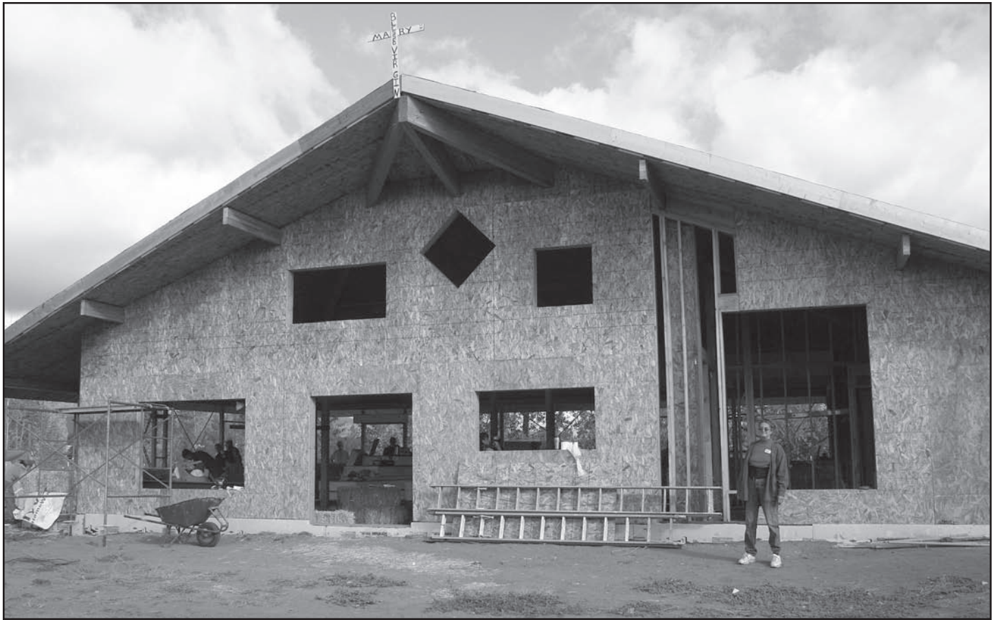
Mary McCracken is building her dream house, which uses a variety of green construction techniques, including straw bale walls.
