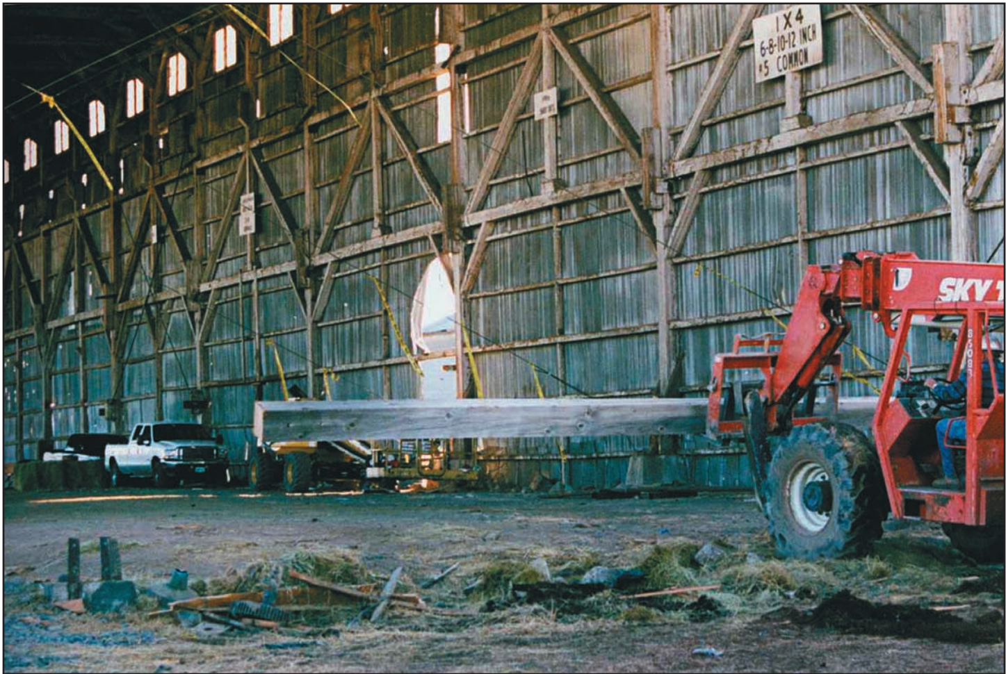
One of the timbers to be salvaged from the L1 shed at the former Edward Hines Lumber Co. mill is moved during dismantling.
